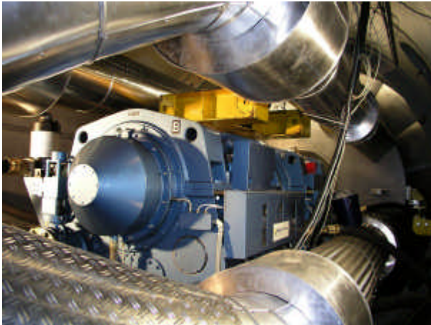
Fig. 6: Water Brake System installed in the Test Cell
